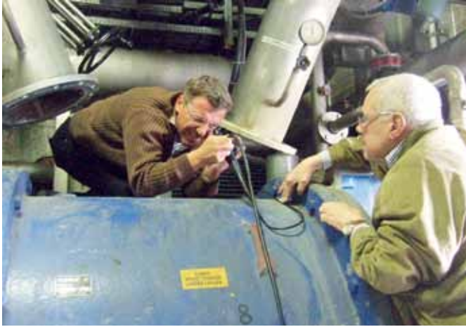
On-site analysis of a vacuum pump by Richter service engineers (here Heinz Heiliger, left and H. F. Laub)
